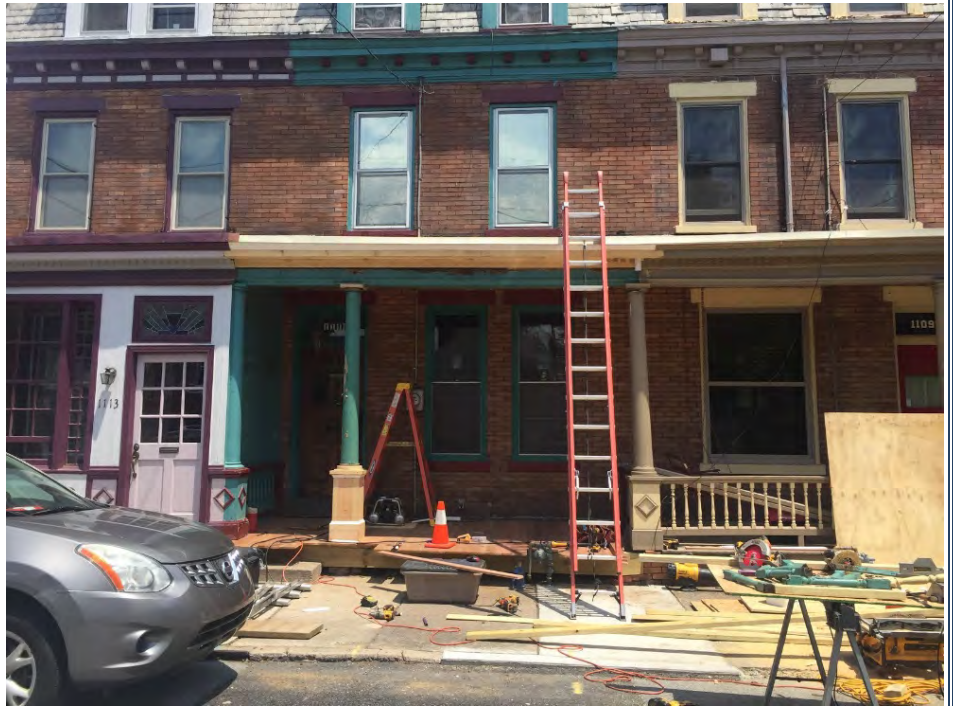
Shown in this photo is an historic Midtown porch undergoing a full in-kind rehabilitation. The new porch will match the original in appearance, material, and texture.
