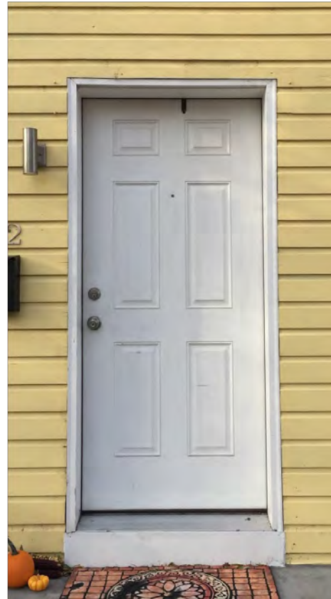
This historic entrance has been severely altered by the removal of its original surround and door. The new steel door is not appropriate replacement.
