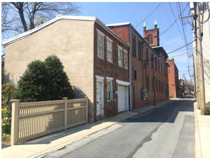
An example of a stucco party wall in Midtown. These walls can be repaired and maintained as needed.
