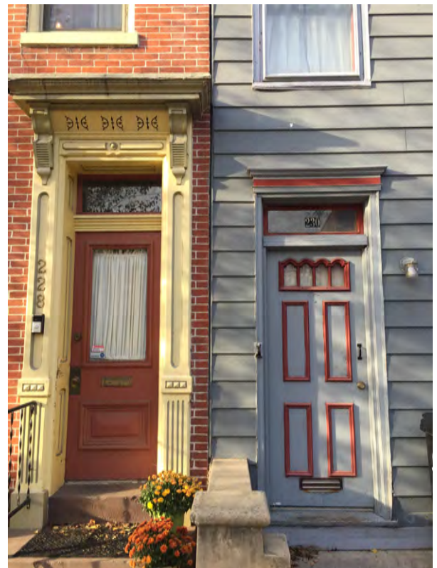
The door and surround on the left has been maintained and preserved whereas the door and surround on the right has been severely altered.
