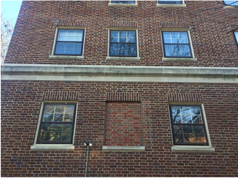
The infill of this historic window opening severely disrupts the rhythm and pattern of the building's exterior.
