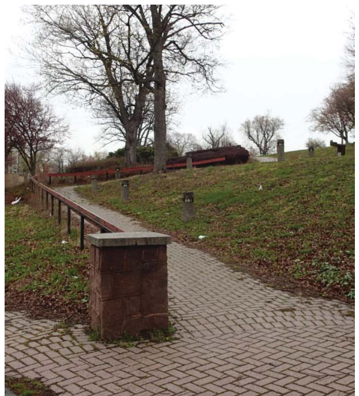
Many of the walkways from the 1990's improvements do not fully conform to today's accessibility standards.
